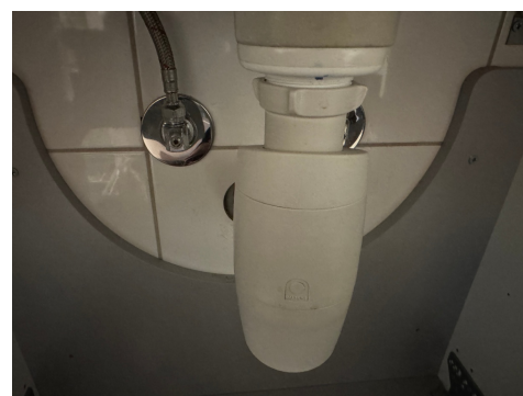
Rørapplegg under servant.
