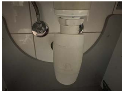
Røropplegg under servant.
