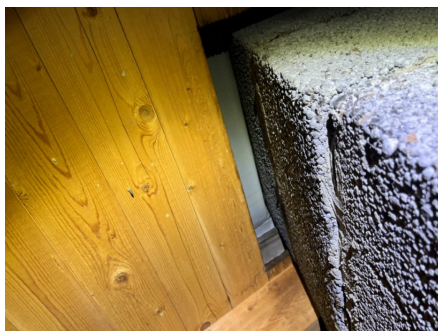
Manglende tetting rundt pipe
