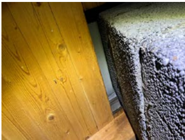
Manglende tetting rundt pipe
