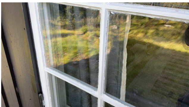
Sprekkdannelse i kitt
