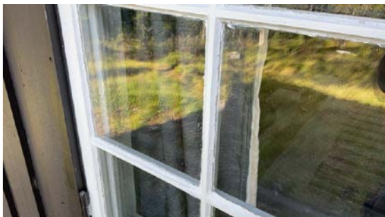
Sprekkdannelse i kitt
