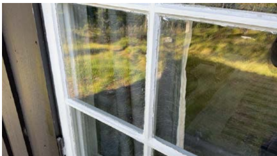
Sprekkdannelse i kitt
