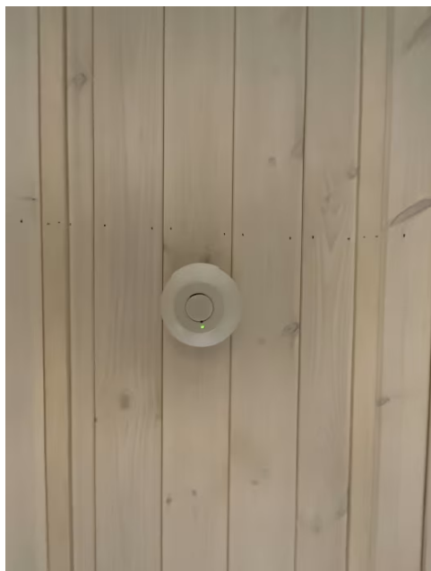
Viser brannmelding montert i himling.
