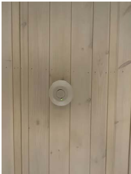
Viser brannmelding montert i himling.
