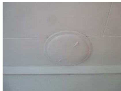
Ventil i himling.
