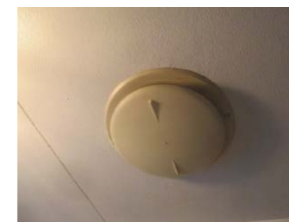
Ventil i himling.
