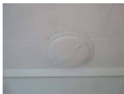
Ventil i himling.
