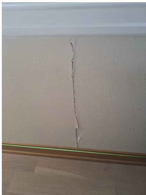
Riss i veggflate.
