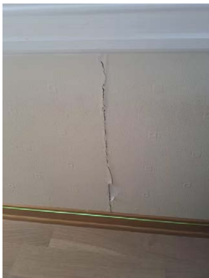
Riss i veggflate.
