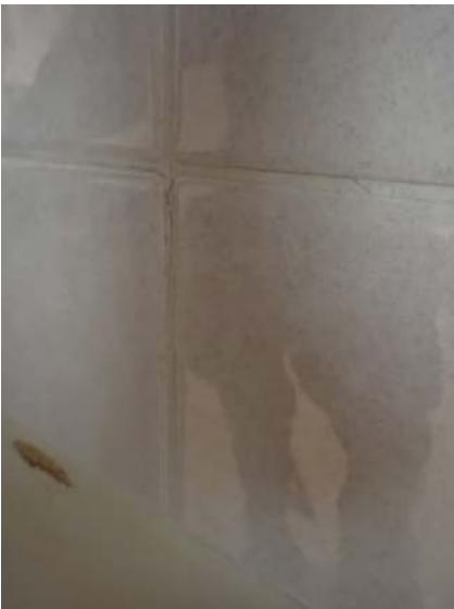
Bom/riss i flis/fuger.
