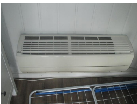
Eldre varmepumpe under trapp.
