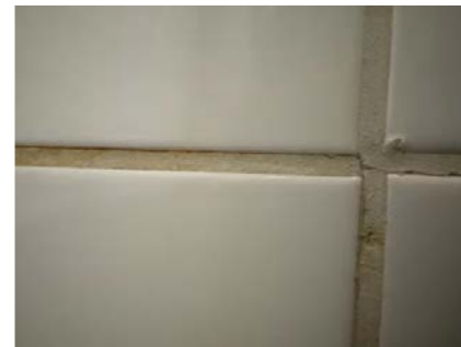
Riss i fuger.
