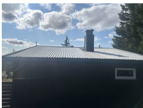
Manglende adkomst for feier.
