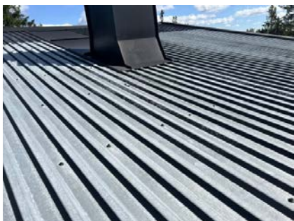
Manglende adkomst for feier.
