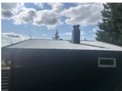
Manglende adkomst for feier.
