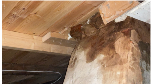
Det lyser inn rundt pipe.
