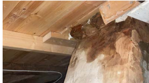
Det lyser inn rundt pipe.
