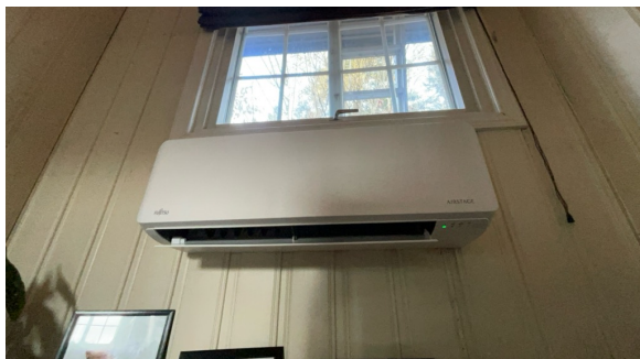
Varmepumpe, innvendig aggregat.
