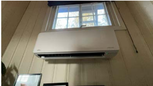
Varmepumpe, innvendig aggregat.
