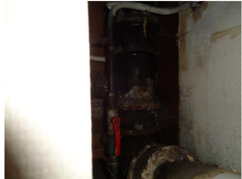
Stoppekran i bod.
