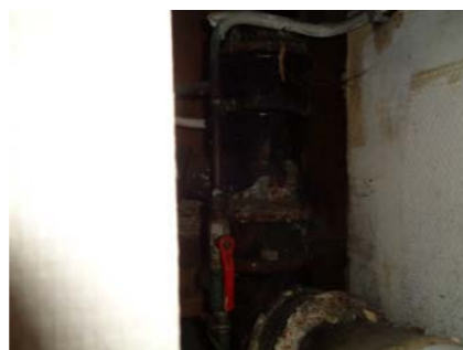
Stoppekran i bod.
