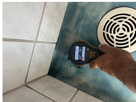
Fukt under belegg
