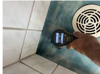
Fukt under belegg
