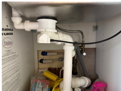
Røropplegg under vask.
