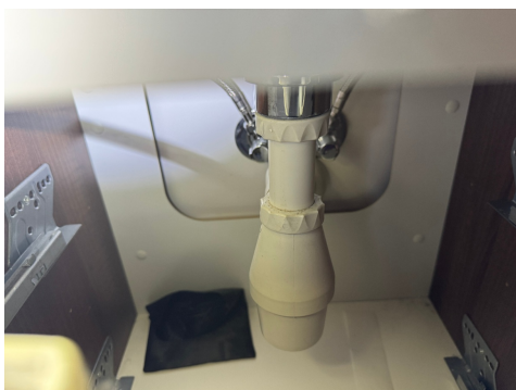
Røropplegg under servant.
