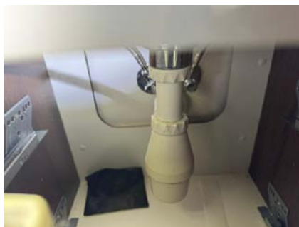
Røropplegg under servant.
