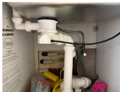
Røropplegg under vask.
