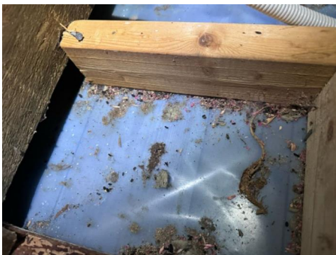
Viser mangelfull isolering.
