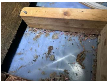
Viser mangelfull isolering.
