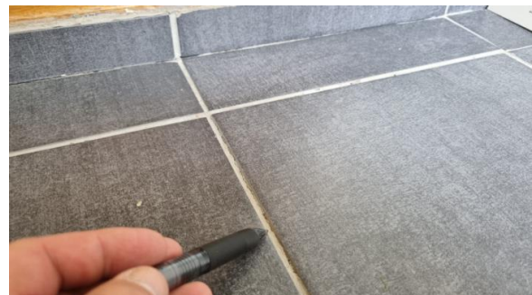
Sprekker/riss i flisfuger.
