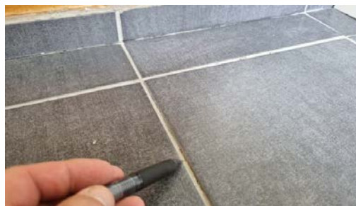
Sprekker/riss i flisfuger.
