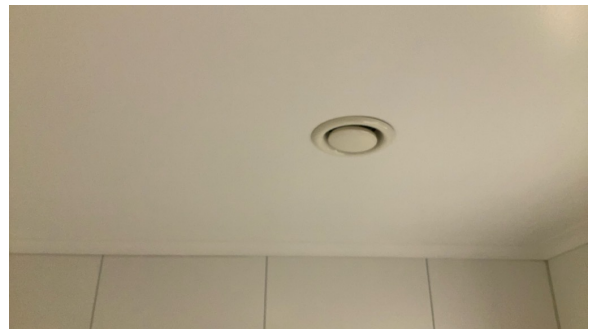
Ventil i himling
