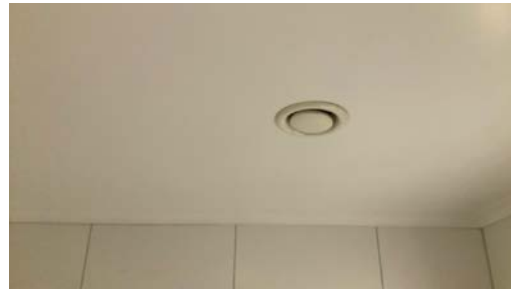
Ventil i himling
