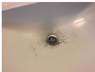
Krakelering i servant.
