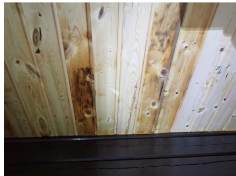
Misfarging i takpanel over veranda.
