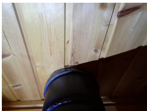
Skjolder i himling.
