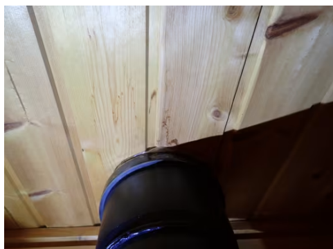
Skjolder i himling.
