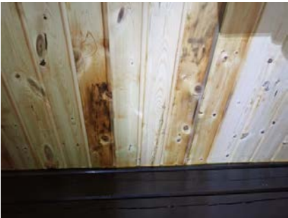
Misfarging i takpanel over veranda.
