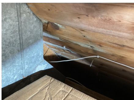
Muggsopp i undertak
