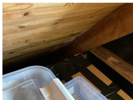
Muggsopp i undertak
