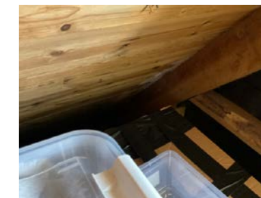
Muggsopp i undertak
