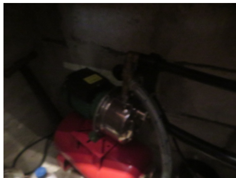
Gammel pumpe under kjøkken.
