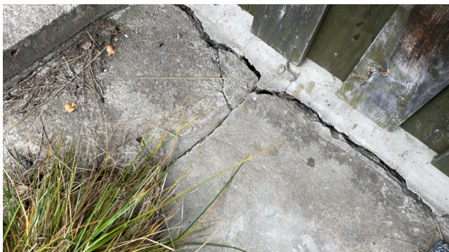
Sprekker i betong
