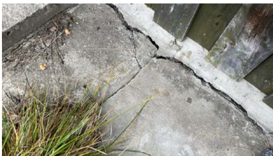
Sprekker i betong
