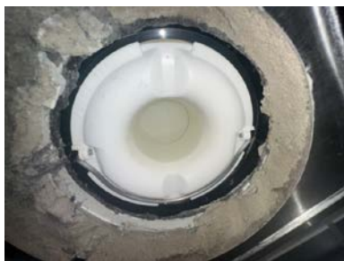
Sluk i plast, plassert under servant
