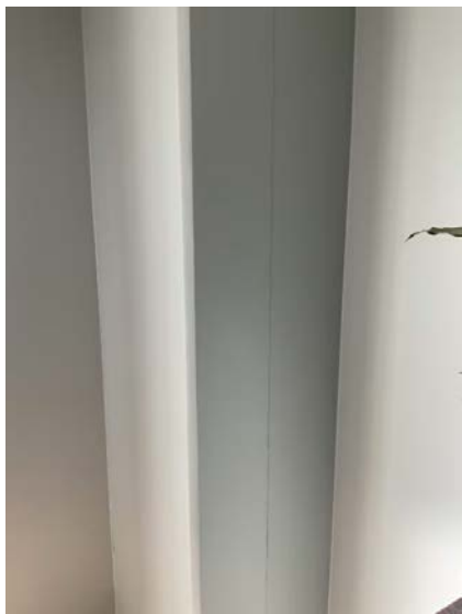
Sprekk i maling.
