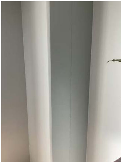
Sprekk i maling.
