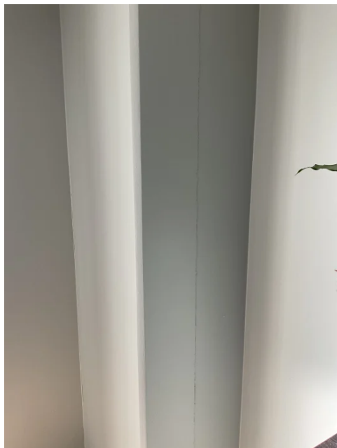
Sprekk i maling.
