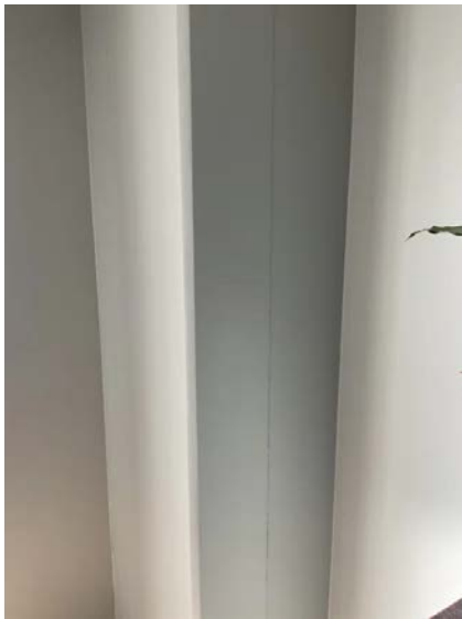
Sprekk i maling.
