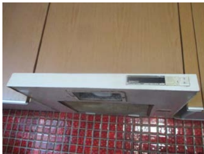
Noe eldre ventilator.
