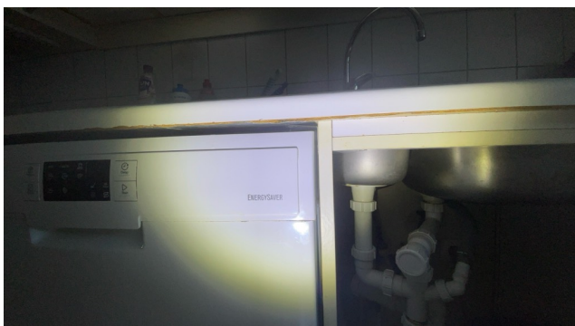
Svelling underkant benkeplate
