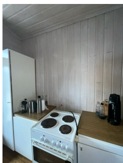
Manglende ventilering over kokesone.
